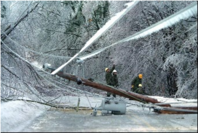
Electric distribution - weather
