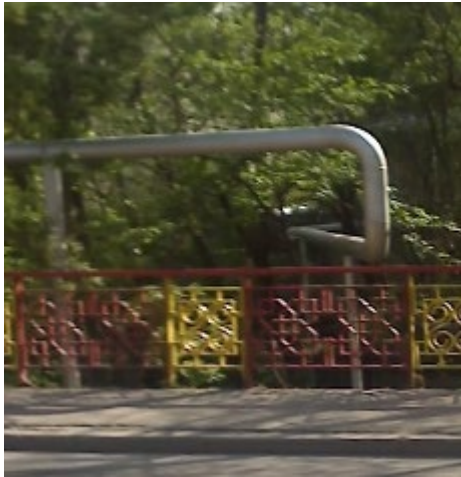
Gas pipes - seismic
